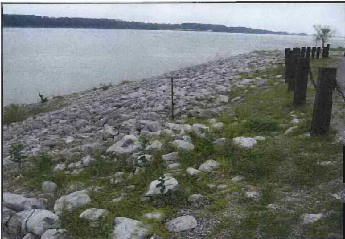
Photograph 2: Facing upstream from the proposed expansion of Schultz Park. Paducah Riverfront Development Phase 1 / Transient Dock. May 14, 2008.
