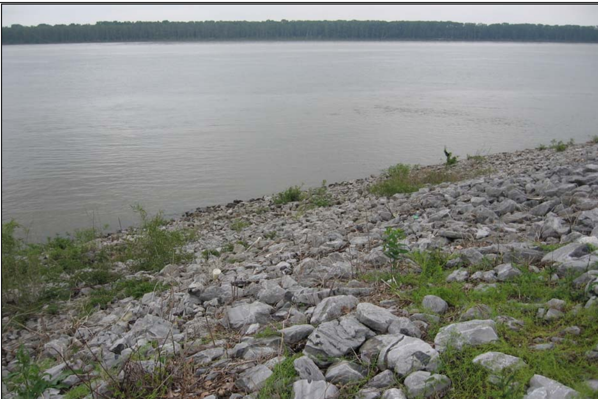
Photograph 4: The majority of the existing riverbank throughout the project area consists of riprap with scattered vegetation. Paducah Riverfront Development Phase 1 / Transient Dock. May 14, 2008.
