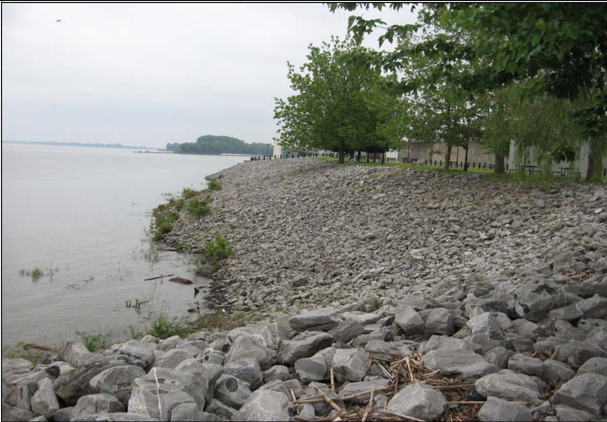
Photograph 3: Facing upstream in the area of the proposed Schultz Park expansion. The existing Schultz Park is located above the riprap bank to the right. Paducah Riverfront Development Phase 1 / Transient Dock. May 14, 2008.
