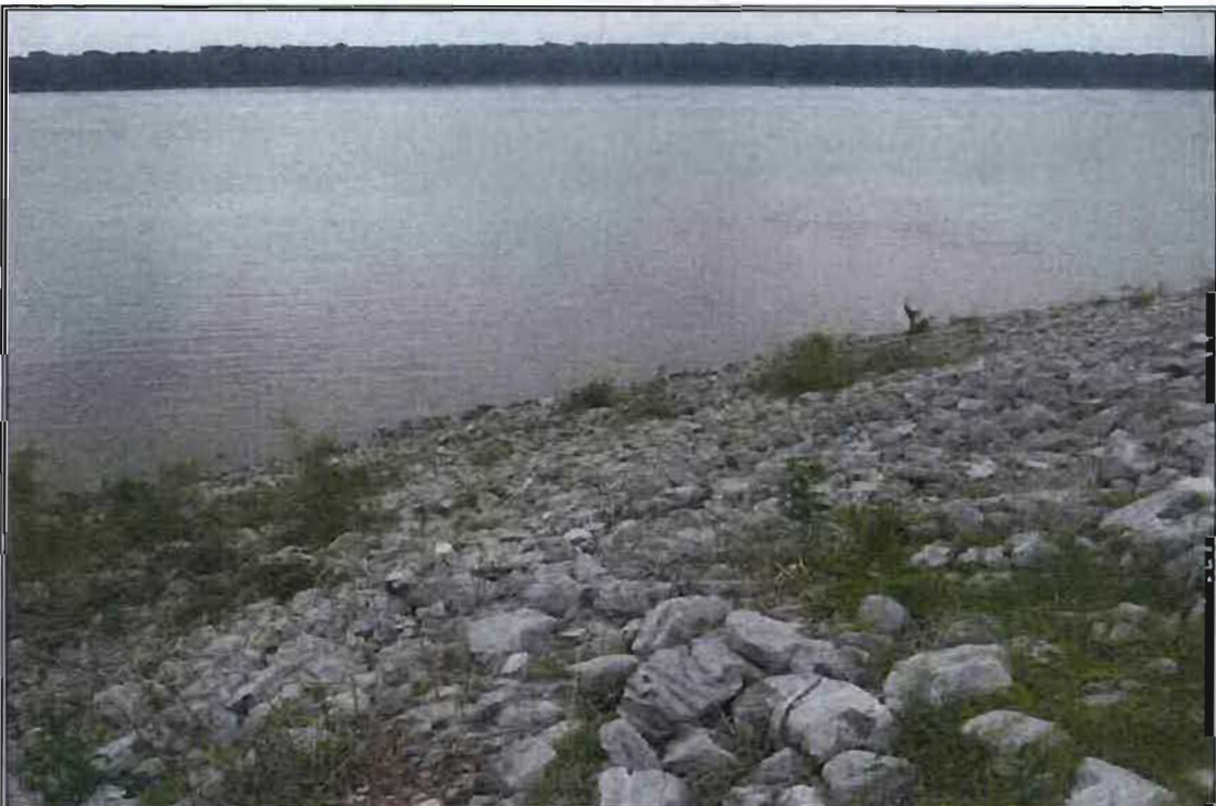
Photograph 4: The majority of the existing riverbank throughout the project area consists of riprap with scattered vegetation. Paducah Riverfront Development Phase 1 / Transient Dock. May 14, 2008.
